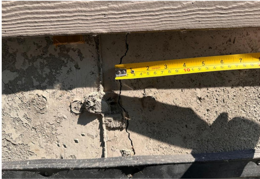
Figure 3: Close up of crack in the concrete foundation
