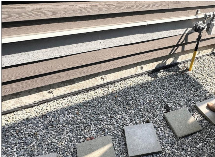
Figure 2: Crack in the concrete foundation
